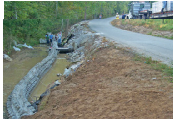
Embankment before project began PHOTO: ARMORTEC
