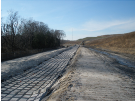
Photo: George and Lynch Inc. The shallow slopes at this site made Cable Concrete a natural choice.
