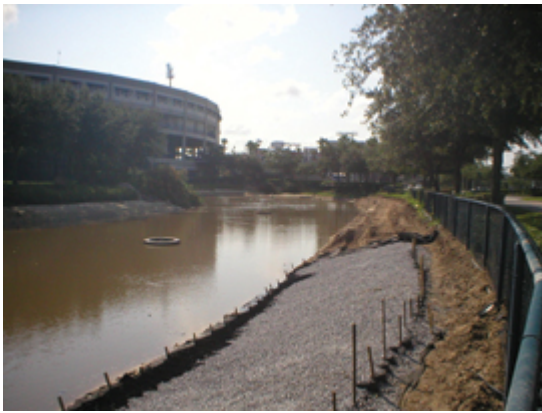
Photo: James Griffin The Legends Field channel during installation of the Geoweb
