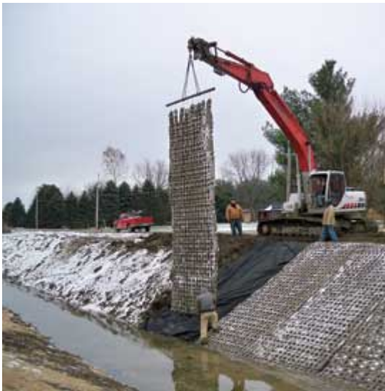
Photo: Charles E. Leser, Madison County The Indiana Department of Environmental Management required articulated concrete block mats for the bridge.
